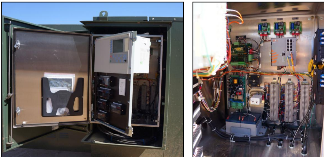
Figure 8: Switch control cabinet with relay, test switches, Ethernet switch, and batteries
