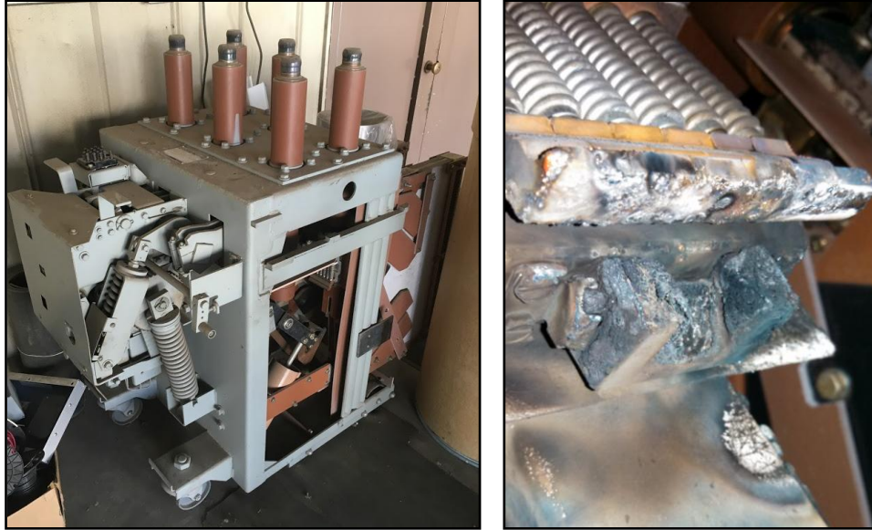
Figure 3: Old main switch with melted contacts
